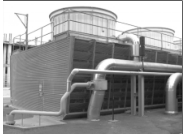
Cooling tower at Sandia's Microelectronics Development Laboratory uses recycled process water for make-up.
