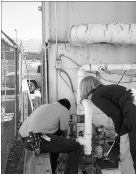
Auditor Christy Smith and facility operations manager examine cooling tower at Amberly Suite Hotel.
