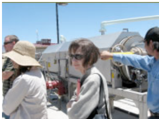
Alice Dareluk (center) of PCR Resources in front of the plant's head works
