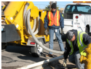
Ruben Archuleta and Rob Paynter check for cleanliness at a fire hydrant water valve
